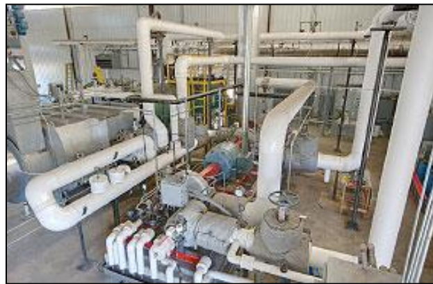
Figure 10 Extraction turbine installed at the Sietsema Gasification Facility
