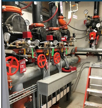
Sprinkler Riser Room
