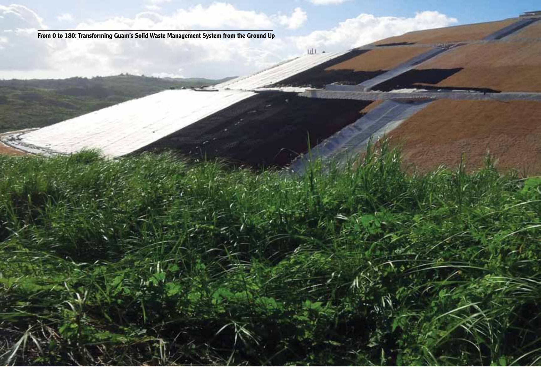
A closure cover of 60 mil LLDPE, geocomposite and geocell is placed over the dump, closed after almost 70 years.
